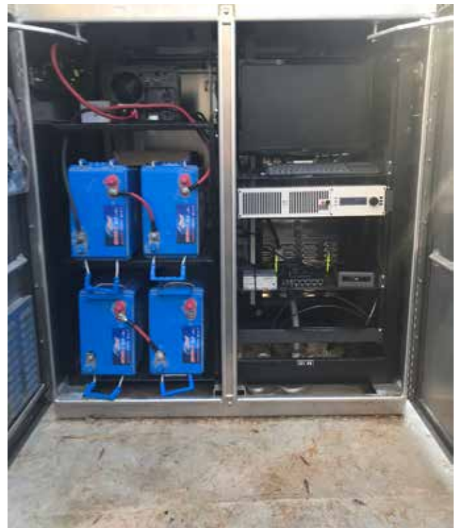
Transmitter cabinet with equipment installed.
